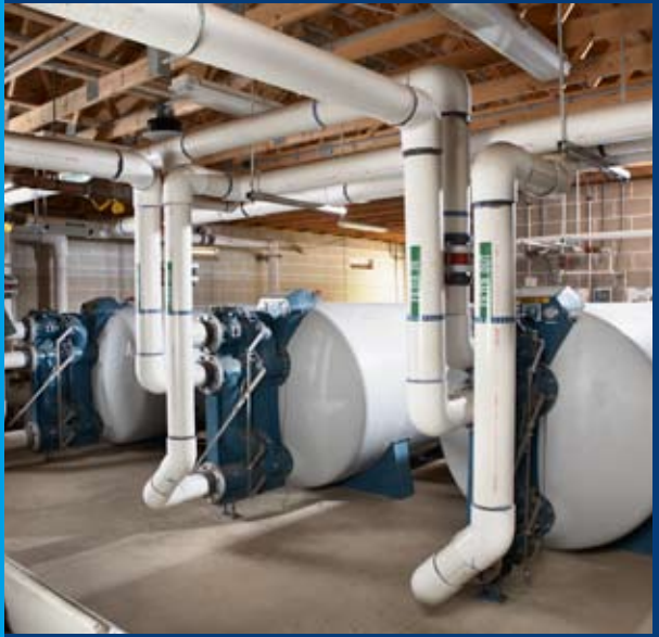
Noelridge Aquatic Center Mechanical Room Cedar Rapids, Iowa
